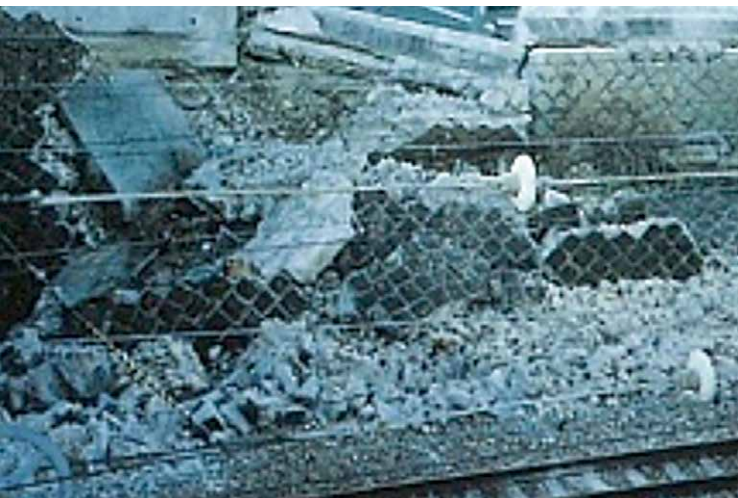
A collapsed retaining wall (Great Hanshin Earthquake in 1995) 1)
