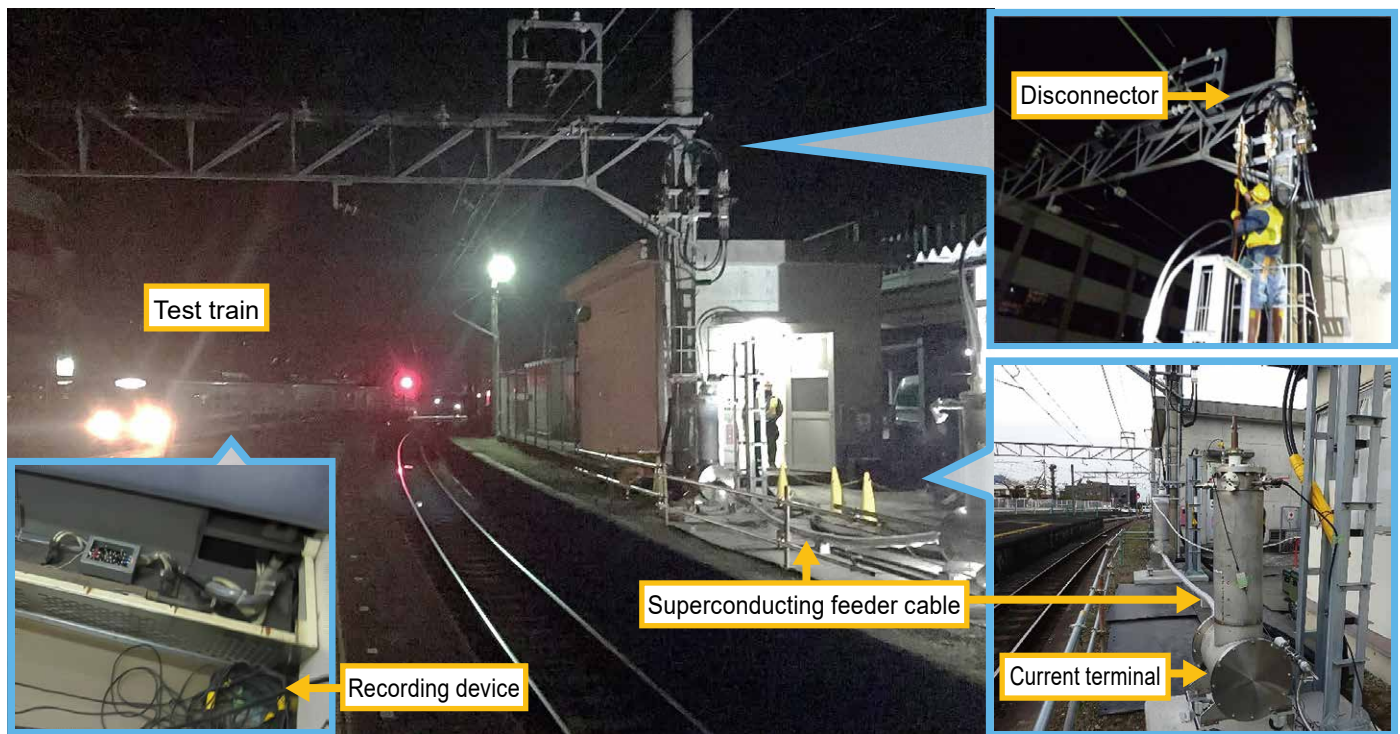
Superconducting feeder cable connected to a track
