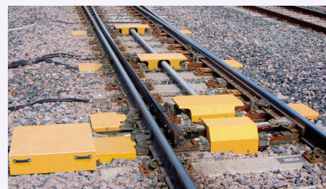
図10 HPSS電気転てつ機(英国) Photo by courtesy of Network Rail.
