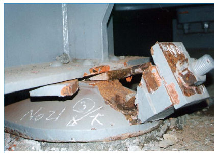
(a) 桁支承の損傷
